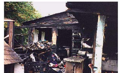
An explosion in a meth lab started the fire that destroyed this building in Thurston County.
