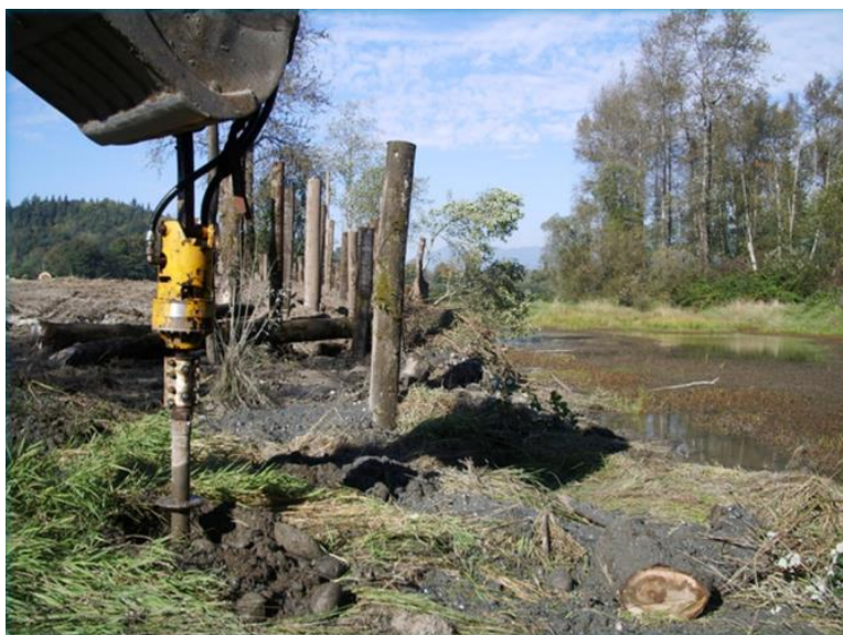
Figure 5 – Example of Flood Fencing Installation along the Skykomish River, WA (Aldrich and DeVries)
